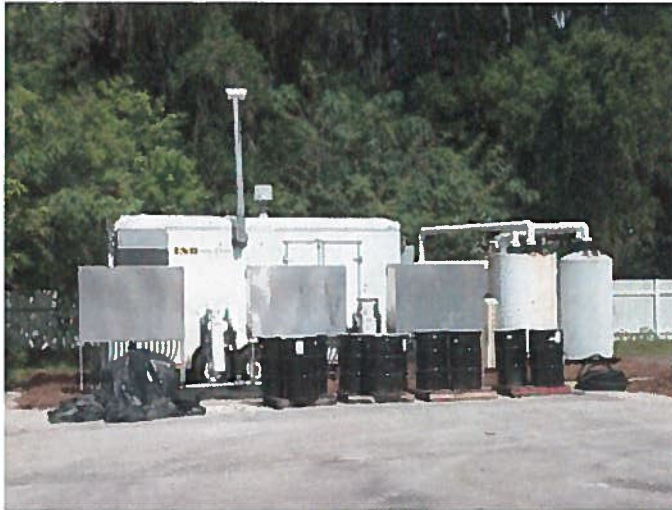
The above trailer at the old Busler Chevy Dealership is designed to filter the contaminated water and put clean water back in the ground.
