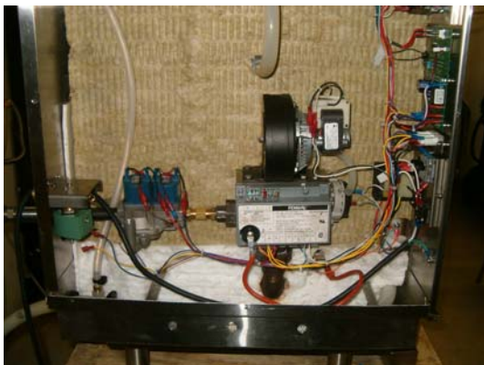
Electronics/hydraulics compartment view.
